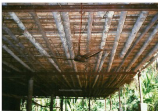
Figure 1. Cattle shed having false ceiling of arecanut stems besides fitted electric fan
