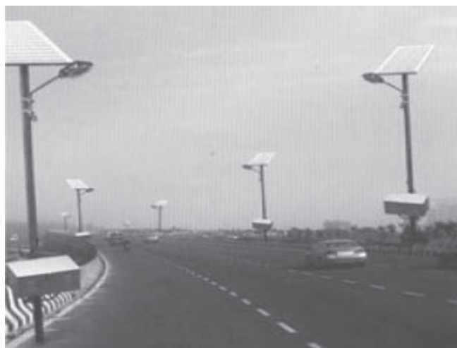
Figure 11: Solar Street light
