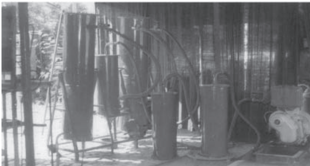
Figure 19: Rice husk gasifier of 10 kW capacities for engine applications (Cost Rs 1.00 lacs)
